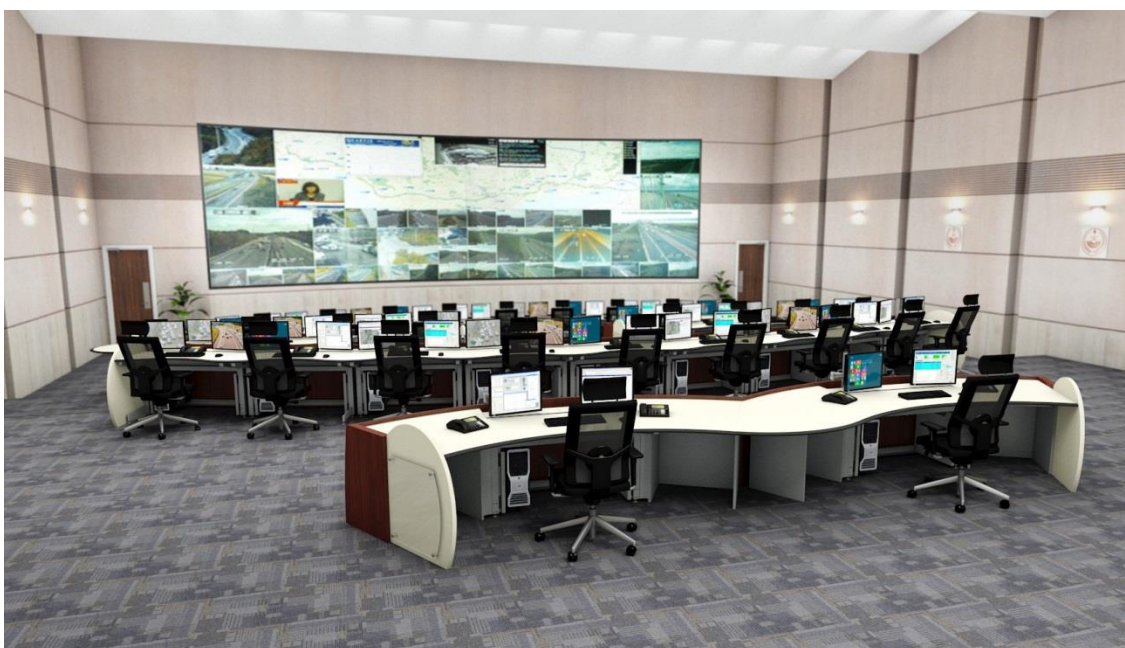
Figure 4: ANTOCC Control Room
